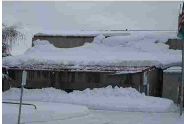
Figure 6.1 Snow sliding. From study of structural failures associated with the winter 2008-2009 snow event in the Spokane/Coeur d'Alene area [SEAW, 2009].
