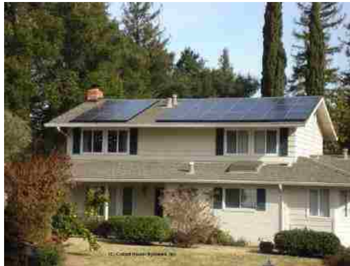
Figure 1.1 PV modules on roof framing systems.
