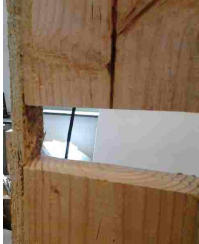
Figure 3.20 Failure of specimen with a glued-and-nailed connection.
