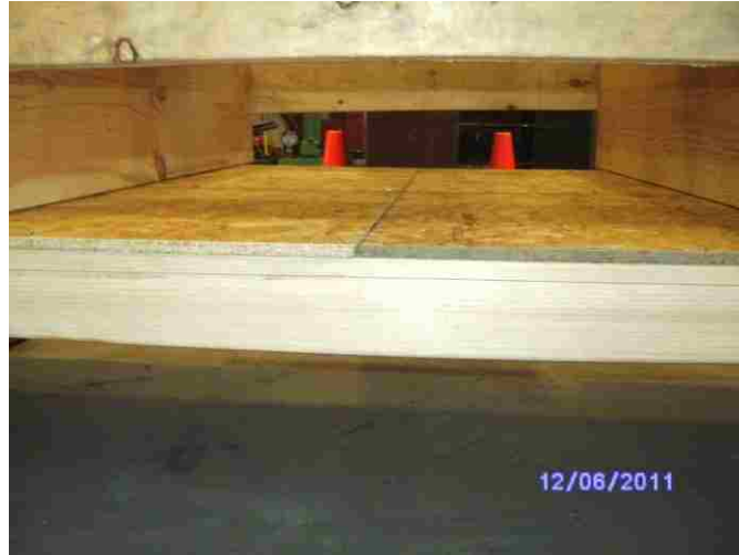
Figure 3.4 Gap at midspan in OSB sheathing.
